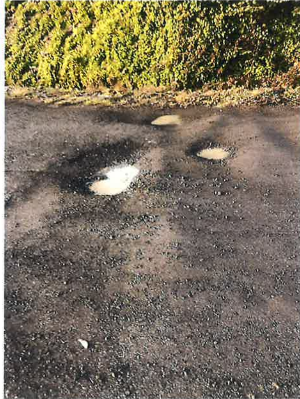
Potholes on Landreth Lane
