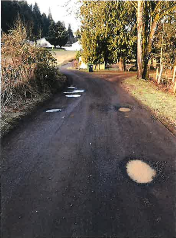
Potholes on Berry Hill Drive
